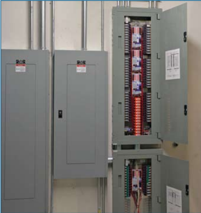
Lighting control system at the Department of Energy's Research Support Facility at the National Renewable Energy Laboratory (Photo courtesy of RNL Design/Frank Doms)
